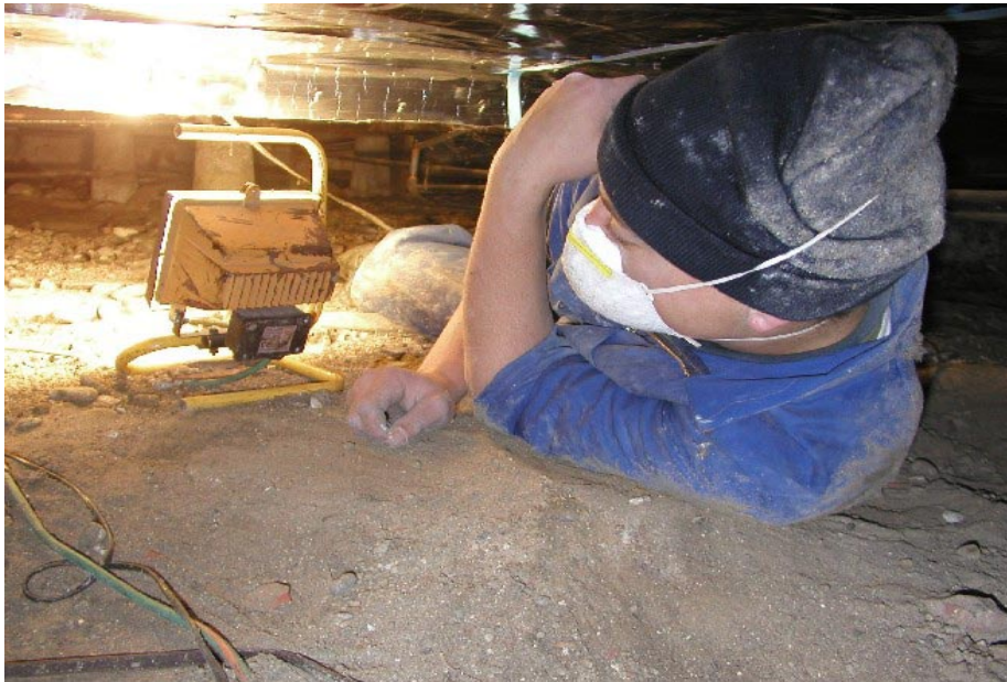
Photo courtesy of CEA, "Hamish Salmon installing insulation in typical tight fitting area"
