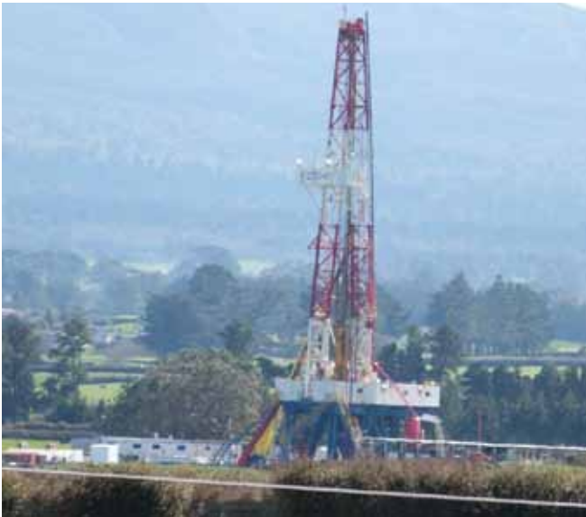
Fig 3- TAG Oil's Cheal C well site and New Zealand Energy Corporation's Copper-Moki well site
